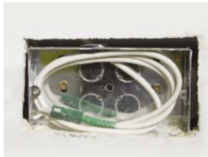
Connectorised end of cable coiled in back box
