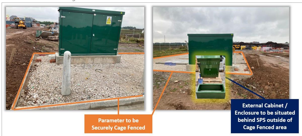
Illustration 2. BDW Trial agreed external cabinet / enclosure onsite location.
