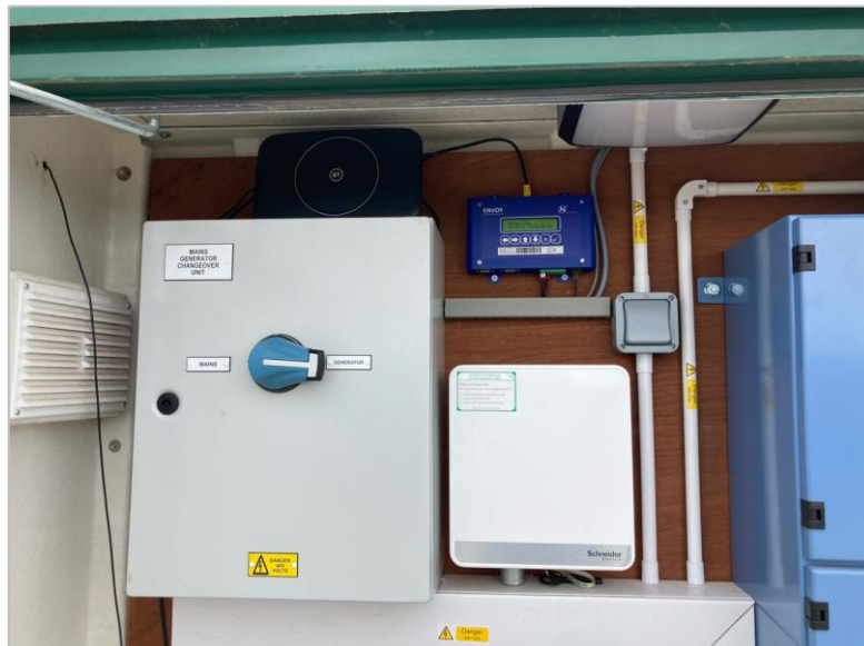
Illustration 6. Nortech: Envoy EV10 installed within Sewage Pump Station
