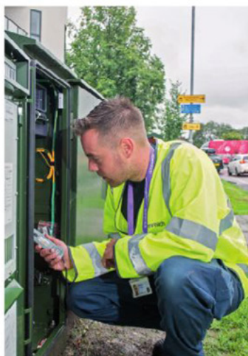
Engineer works on a Gfast side pod
